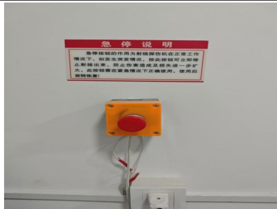
图3-11 探伤室内急停按钮
